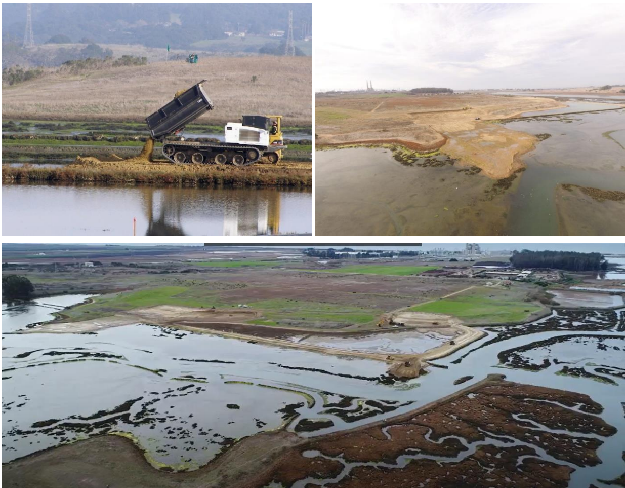
Figure 5.2 Elkhorn Slough Tidal Marsh Restoration Project – South of San Francisco Bay (California)
